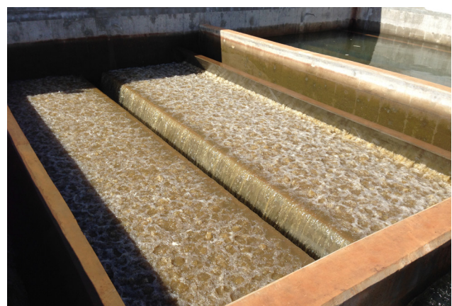
Filter in backwash
